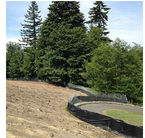
Erosion control features to prevent water quality issues during construction of the Sammamish Community and Aquatic Center
