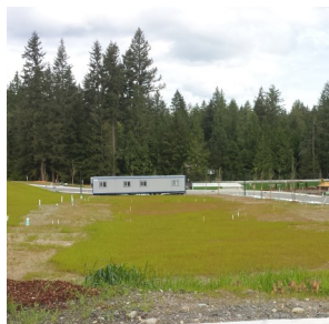
Example of new development under construction. City staff review permits for compliance with stormwater codes and standards, and conduct construction site inspections.
