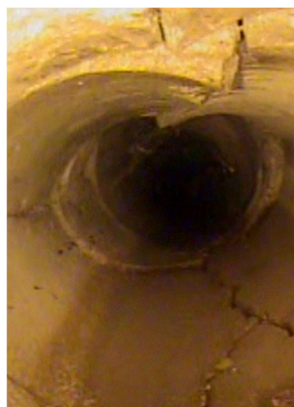
FIGURE 2. EXAMPLE PHOTO FROM VIDEO SCREENING OF PIPE CONDITION (CITY OF NEWCASTLE S-38 PROGRAM WEBSITE)
