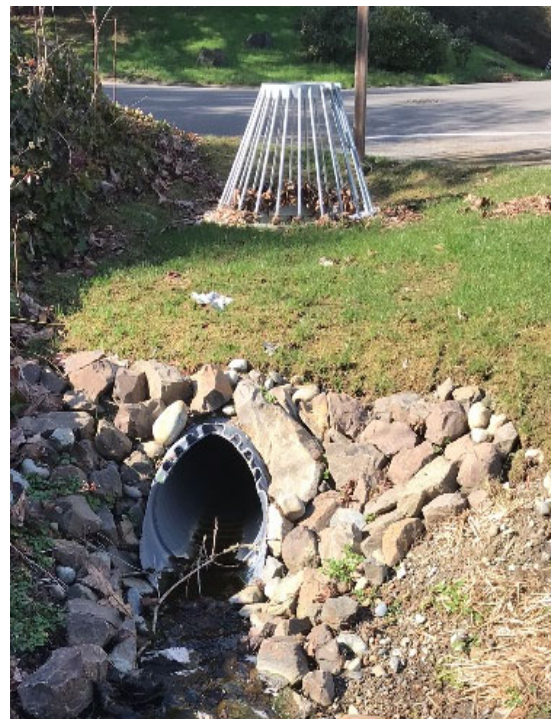
FIGURE 1. NEW CATCH BASIN INSTALLATION AT NE 22ND ST AND 229TH AVE NE
